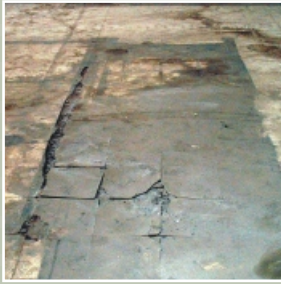
Remove and Repair
